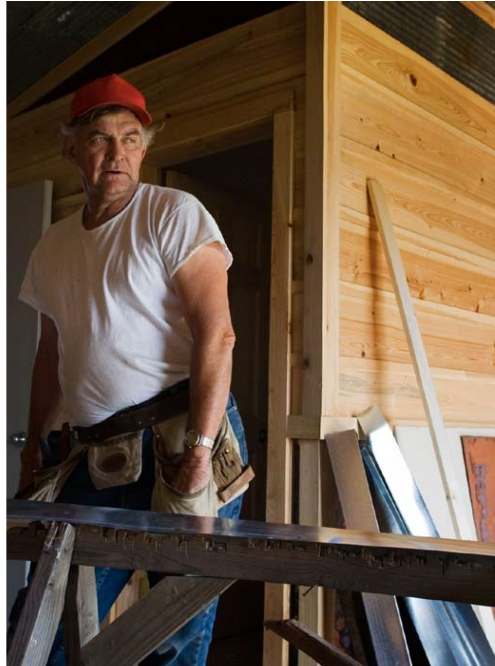
Carpenter Gary Gist at work outside of Clarksdale, Mississippi., 2007; PHOTO BY: DL Anderson
